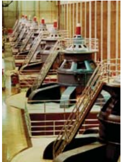
A series of hydels generator.
