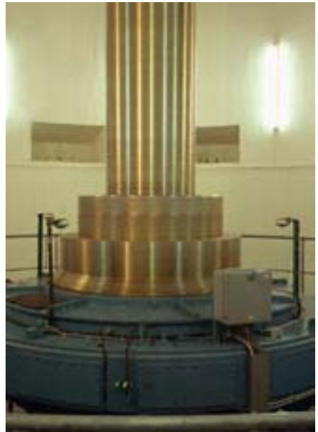
A big hydel generator. Governors are used to control the supply of working fluid (water in hydel generators).
